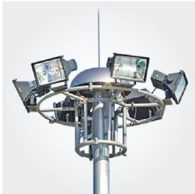
2. HIGH MAST POLE
